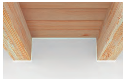
Internal expansion joints
