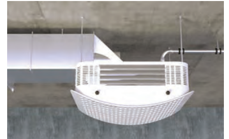
Air conditioning units
