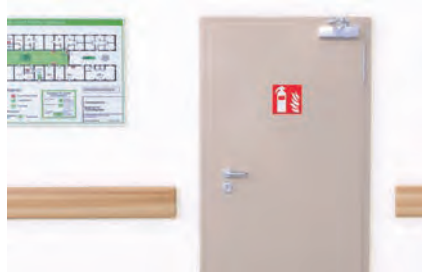
Fire protection doors
