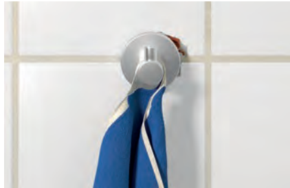
Repairing damaged drill holes
